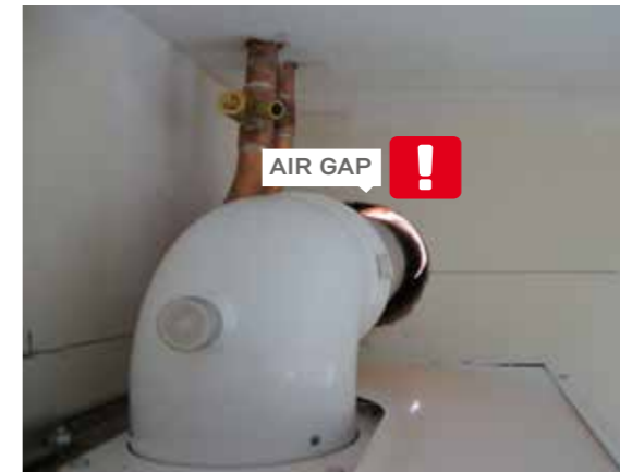
BOILER FLUE NOT SEALED
