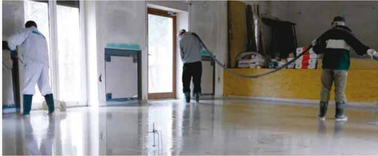
Machine application of the fast-setting anhydrite-based screeds is a perfect solution for large surfaces (over 15 m 2 )
